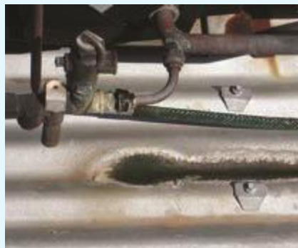
Figure 1: Bi-metallic corrosion caused by ‘copper-rich’ water run-off
